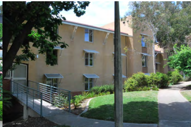
Figure 8: The western face of the building including access ramp and landscaping. (Source: ANU Heritage Office 2011)
