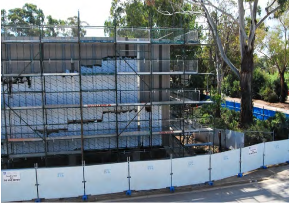
Figure 9: View of the construction of the HPCF from JCSMR. (Source: ANU Heritage Office 2012)
