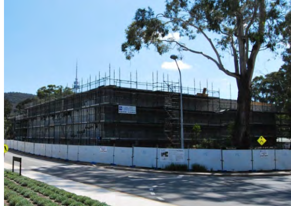
Figure 10: View of the construction of the HPCF from corner of Garran Road and Ward Road. (Source: ANU Heritage Office 2012)
